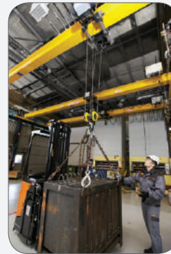
Example of an Overhead Travelling Crane
